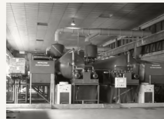
Autoclave treatment station - Moulton production site (14)
